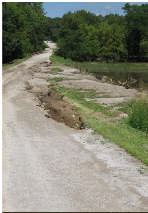
Linn County Flood Damage in August 2009 Photo Source: Linn County Planning and Development
